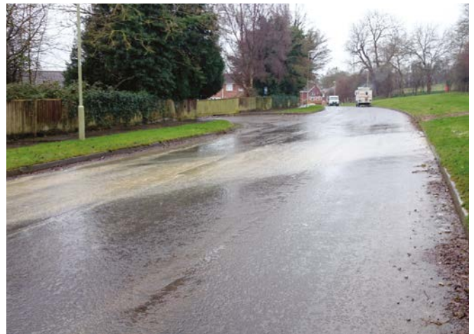
Evidence of rain water run-off leading to flooding from high ground in North Alton across Gilbert White Way
