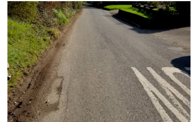
Kerb encroachment and damage to verge
