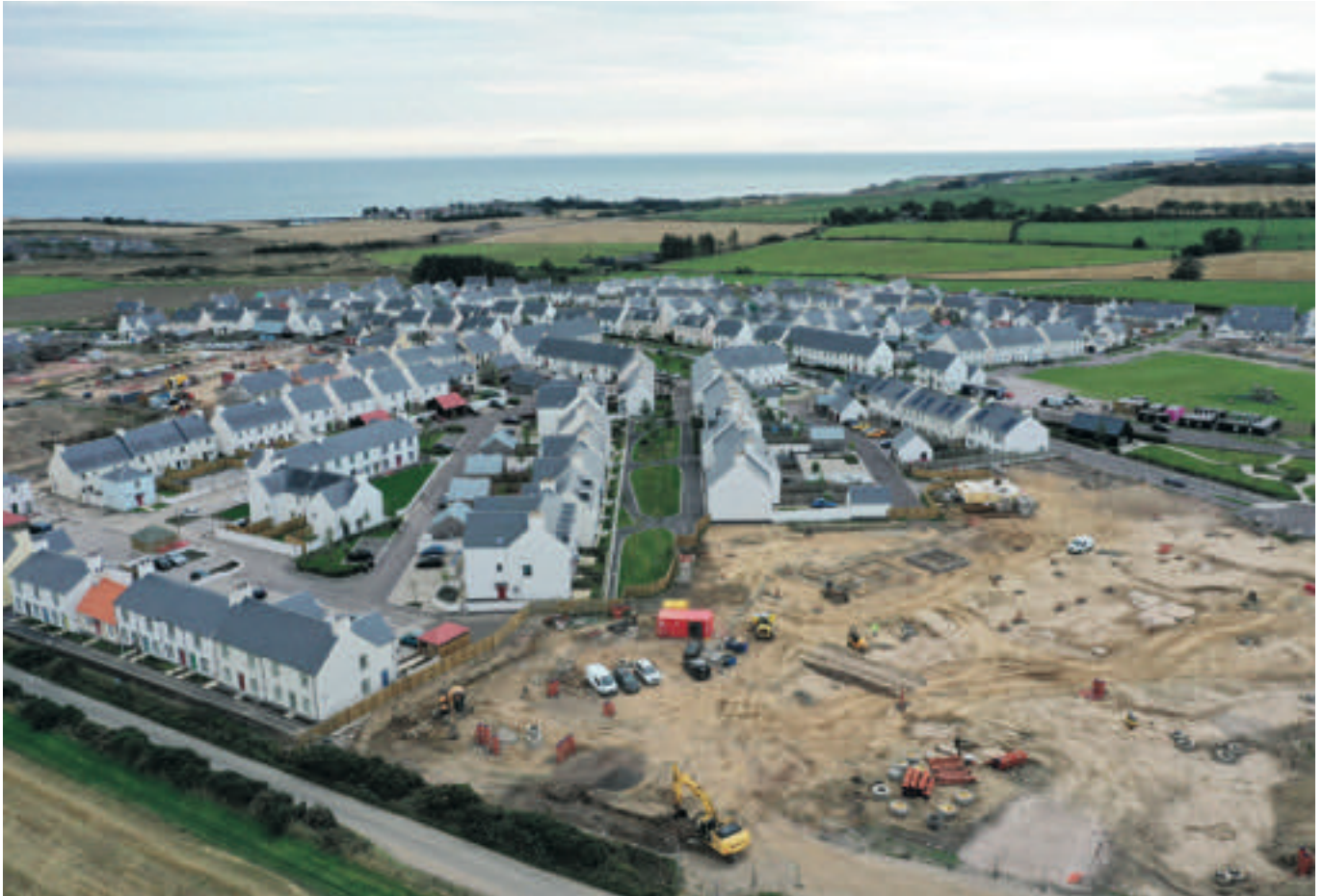
The first phase at Chapelton comprises a range of market and affordable homes inspired by the local vernacular.
